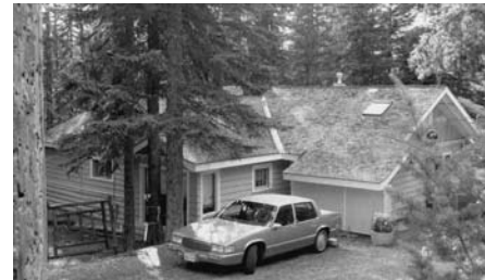
This home's close proximity to combustibles, unrated wood shakes and vinyl siding creates an opportunity for fire to spread easily.
